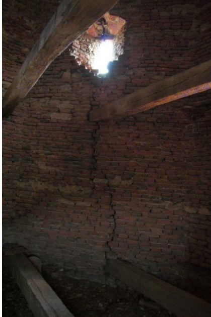
Abb. 37 – Chor, Wehrgeschoss, Riss
